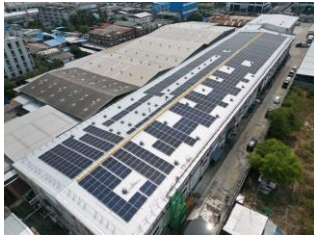
Solar panels (Subsidiary in Thailand)
