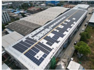
Solar panels (Subsidiary in Thailand)
