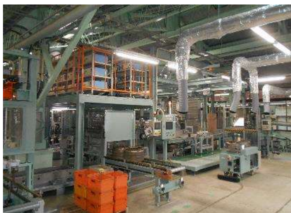
Renewal of in-house plating equipment to improve plating quality and enhance production of screw products
